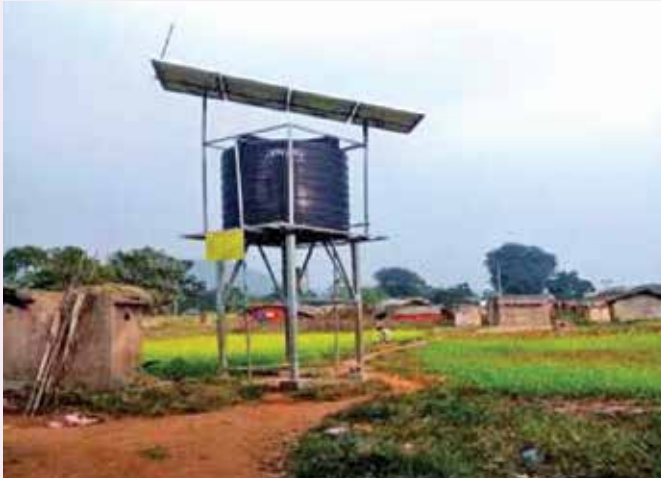
Drinking Water facility under MGNREGA at Katakoli VSS, Keonjhar DMU
