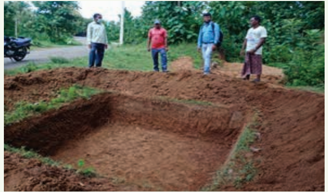
Earthen Compost Pit support to farmers at Dabri VSS through convergence with MGNREGS, Khariar Division
