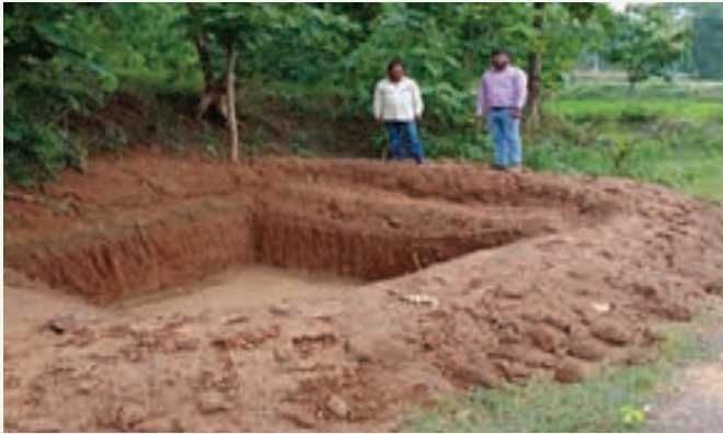
Earthen Compost Pit support to farmers at Kodaldunguri VSS through convergence with MGNREGS, Khariar Division
