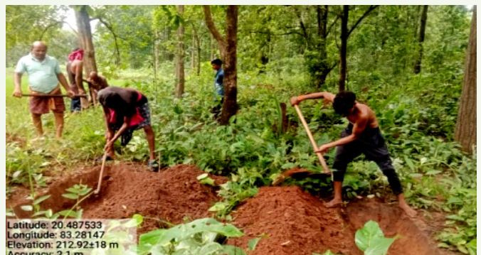
SMC maintenance work at Suliamal VSS under Sainitala Range, Bolangir Forest Division
