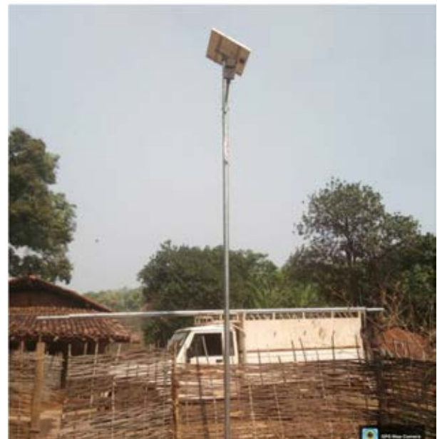
Solar street light in villages
